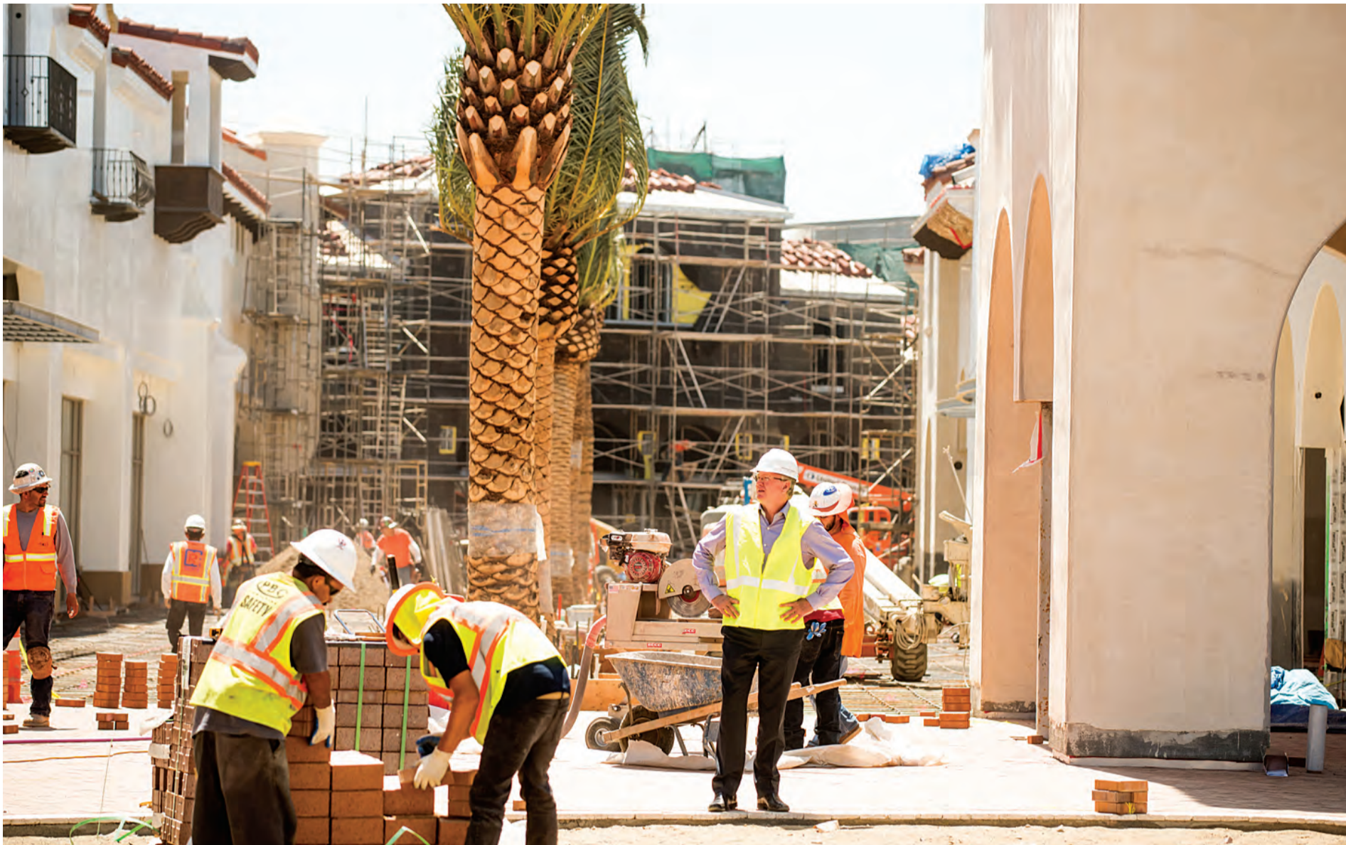
Craig Realty Group Managing Partner Steve Craig surveys construction progress in mid-July.
