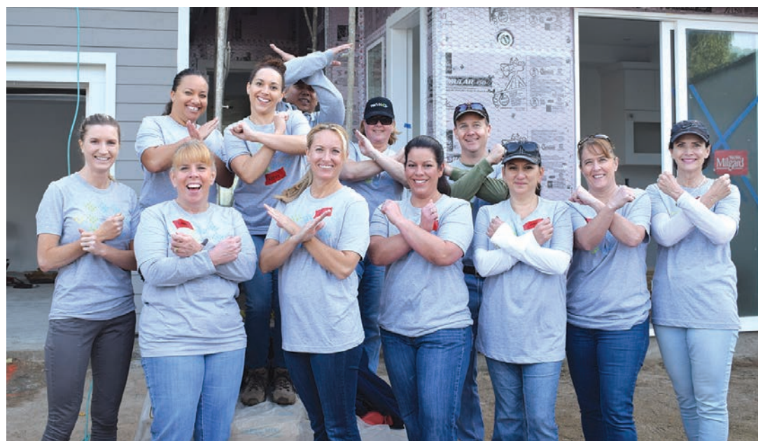
Ten-X employees traded their smartphones for hammers during a Team Build Day where they helped build affordable Habitat for Humanity of Orange County homes.
